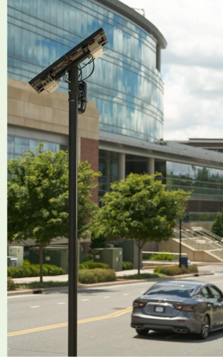
Solar & Flock Pole
